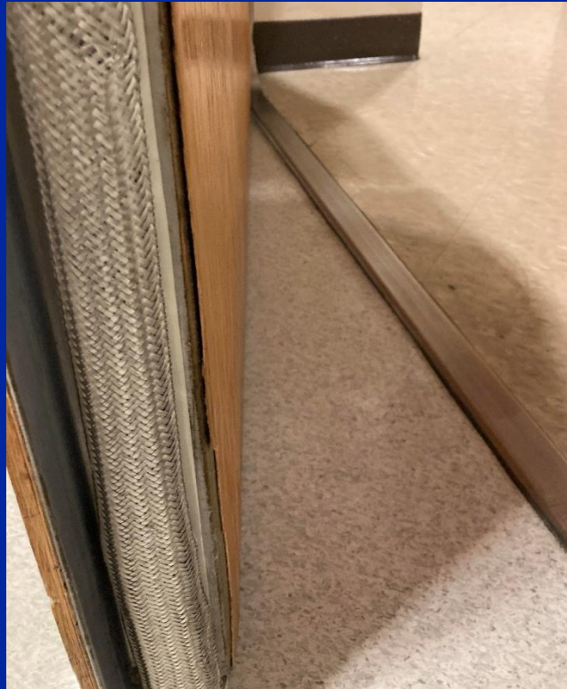
Metal seals around doors
